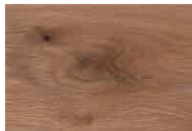
CHECK: A lengthwise opening on the face of the board resulting from rapid or faulty drying.
