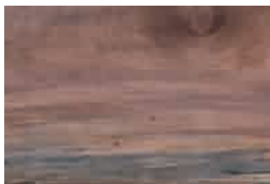
DECAY OR ROT: The breaking down of the wood substance by fungi. The discoloration of the sapwood indicates the initial evidence of decay.
